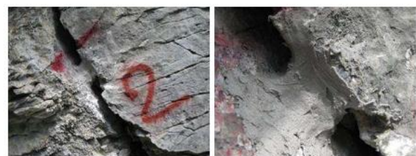
No 2A Installation Date: May 2012 (3rd bi-annual inspection by GEOTEST _ installation by Greek Alpinists)
